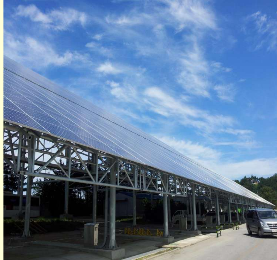
Young Dong Power Plant (1 MW)
